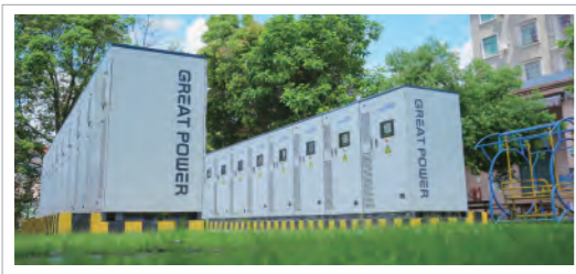
Guangdong Yunfu Xianfeng Stainless Steel Products Co., Ltd. 4.3MWh Energy Storage Project
