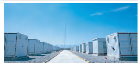
Jimusaer 150MWh Project
