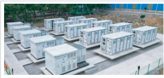
Henan Jinma Energy Co., Ltd. 34.4MWh Energy Storage Project
