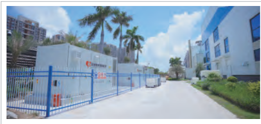
Zhuhai Great Power Production 29.77MWh Project
