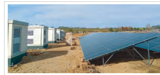
Germany 16.77MWh Containerized Energy Storage Project
