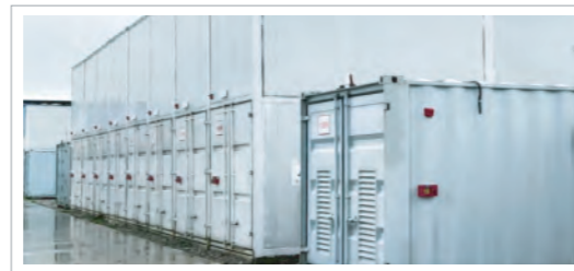
State-Owned Shipyard 100MWh Energy Storage Station Project
