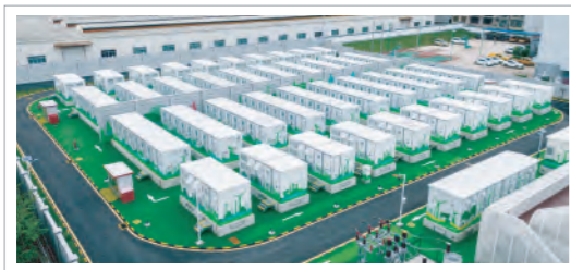
Nanning 100MWh Energy Storage Project
