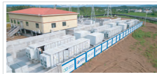
Ji'an 15MWh Agro-Photovoltaic Complementary Project
