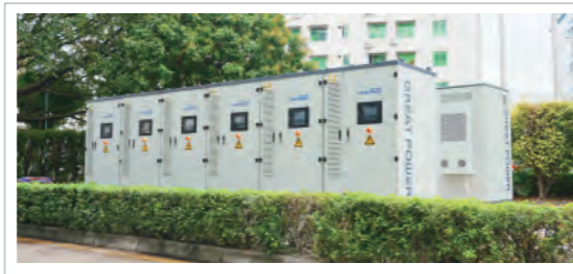
Guangzhou Production 7.33MWh Project
