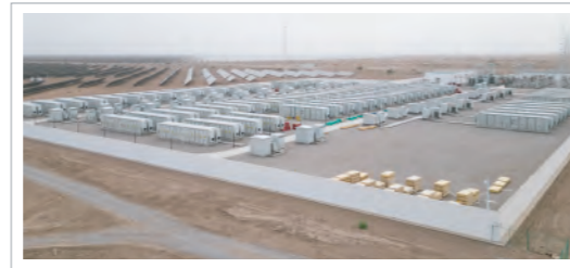
Bachu 140MWh Agro-Photovoltaic Complementary Project
