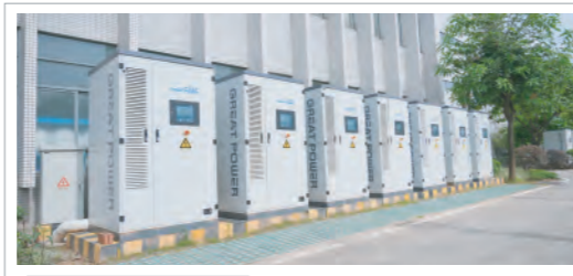
Guangzhou Weili Medical Equipment Co., Ltd. 7.95MWh Project
