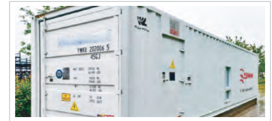
Croatia 17MWh Photovoltaic and Storage Complementary Project
