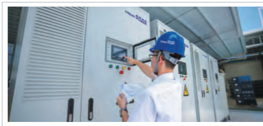
Guangzhou Xinli 2.33MWh Project
