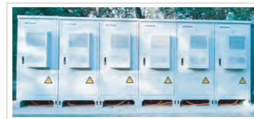
India 2MWh High-Grid Photovoltaic Storage Project
