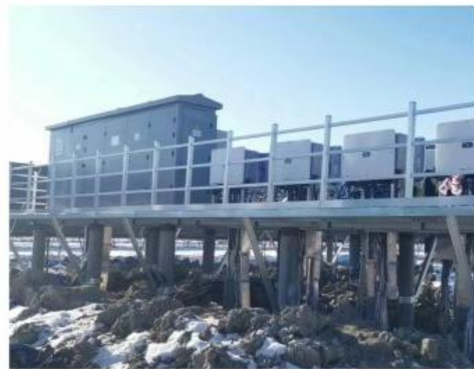
国家光伏、储能实证实验平台项目 National Photovoltaic and Energy Storage Demonstration and Testing Platform Project
