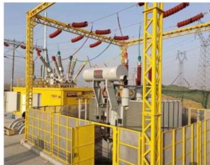
河北雄安新区移动变电站项目 Mobile Substation Project in Hebei Xiong'an New District
