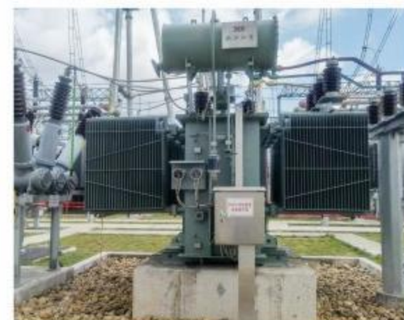
南网±800千伏超高压 穗东换流站扩建项目 China Southern Power Grid ±800kV Ultra-high Voltage Sui Dong Converter Station Expansion Project
