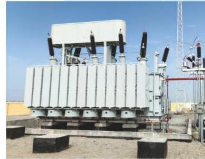
国电投洛浦县220kV光伏汇集站 SPIC 220kV Photovoltaic Gathering Station in Luopu County
