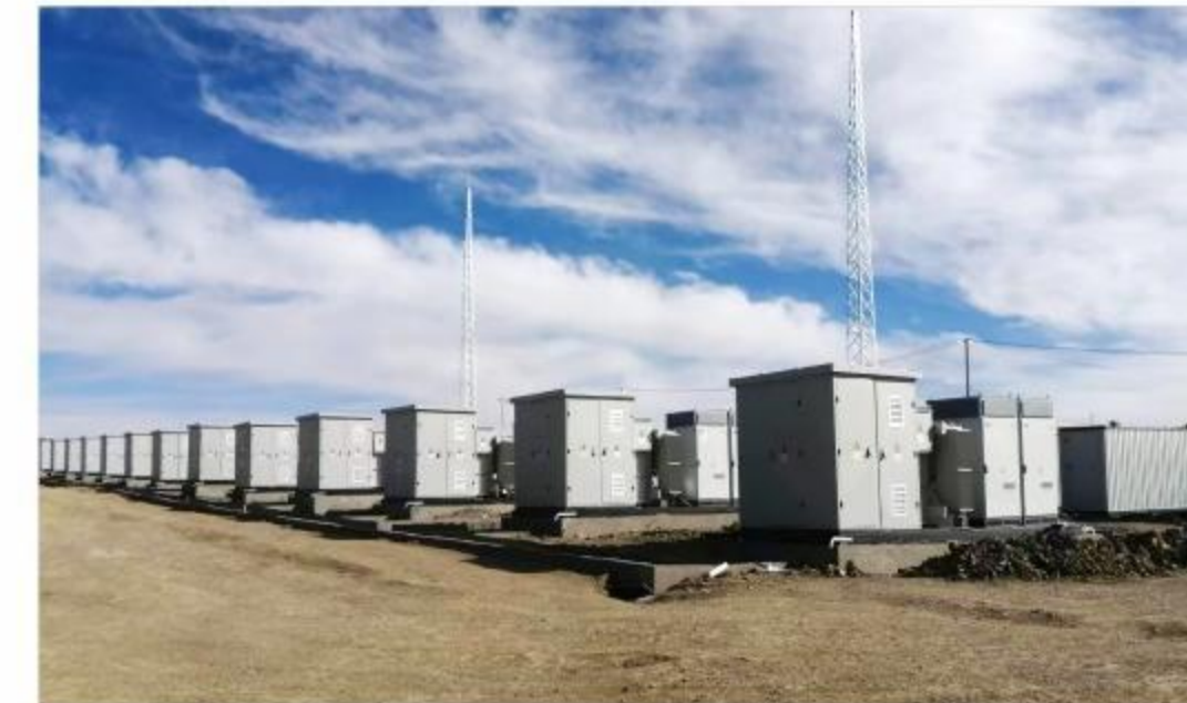
西藏华电那曲光储电站储能一体机项目 Tibet Huadian Naqu Solar-Storage Power Station Energy Storage Integrated Skid Project
