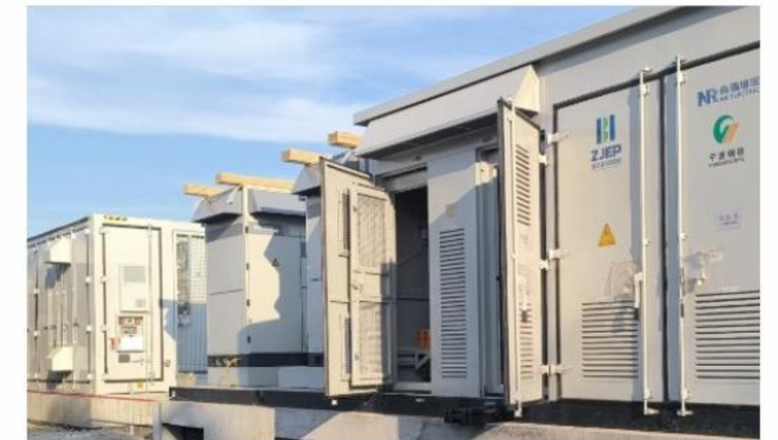
宁波钢铁储能项目50MW/100MWh Ningbo Steel Energy Storage Project 50MW/100MWh
