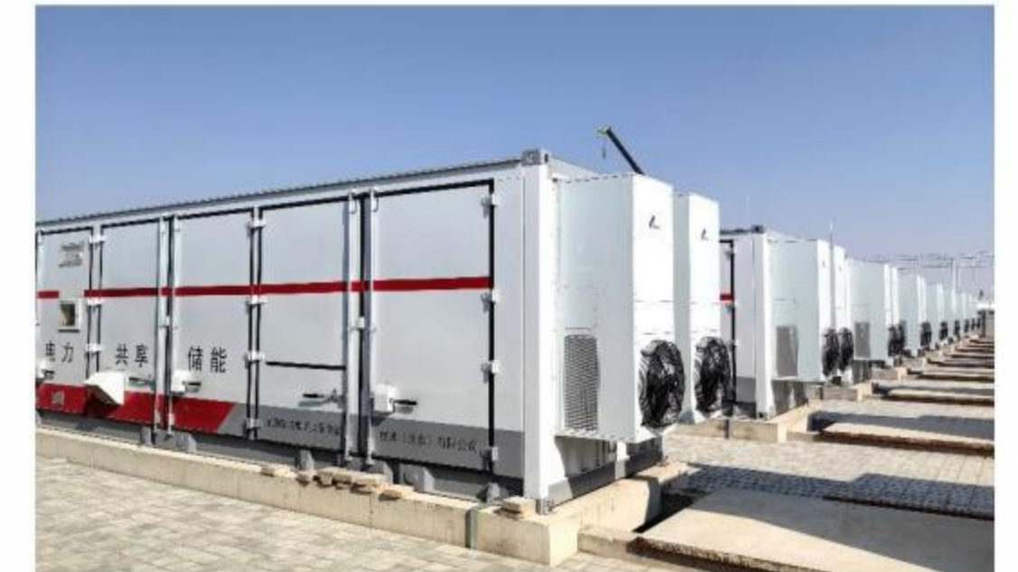
宁夏龙源储能项目100MW/200MWh Ningxia Longyuan Energy Storage Project 100MW/200MWh
